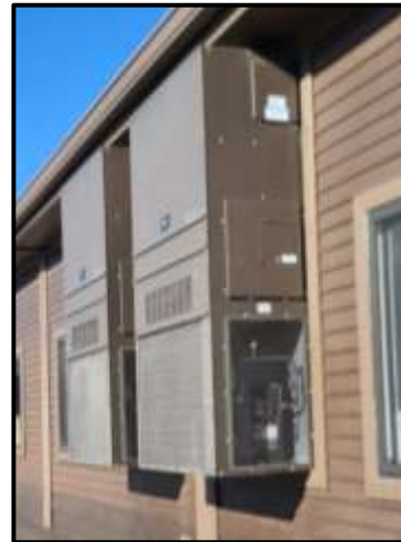
Figure 5: Double Mechanical Unit on Southeast Addition Exterior
