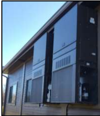
Figure 3: Mechanical Units on Northwest Addition Exterior
