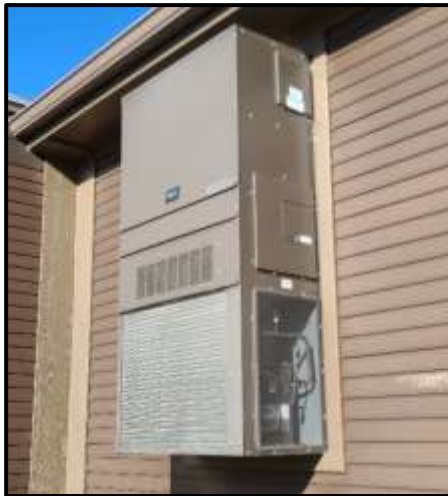
Figure 4: Single Mechanical Unit on Southeast Addition Exterior
