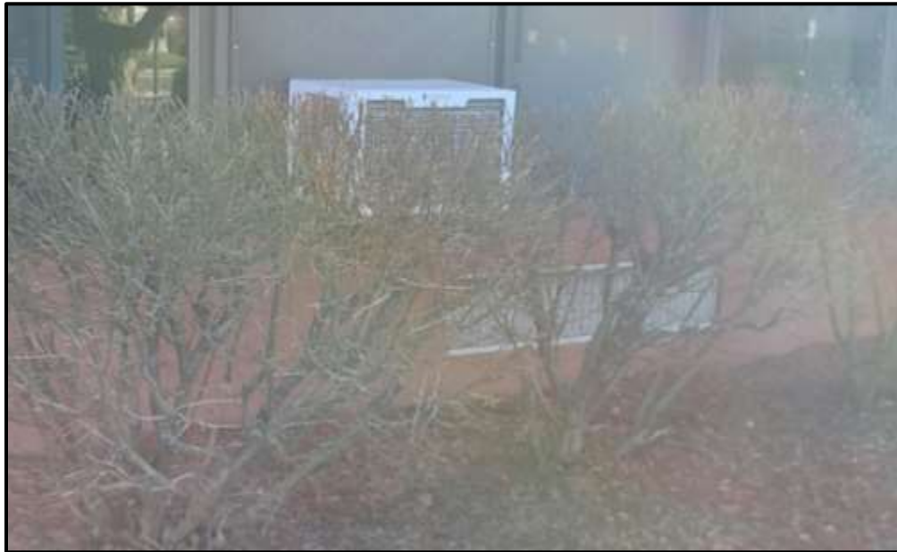
Figure 1: Measured Air Conditioning Unit in Courtyard
