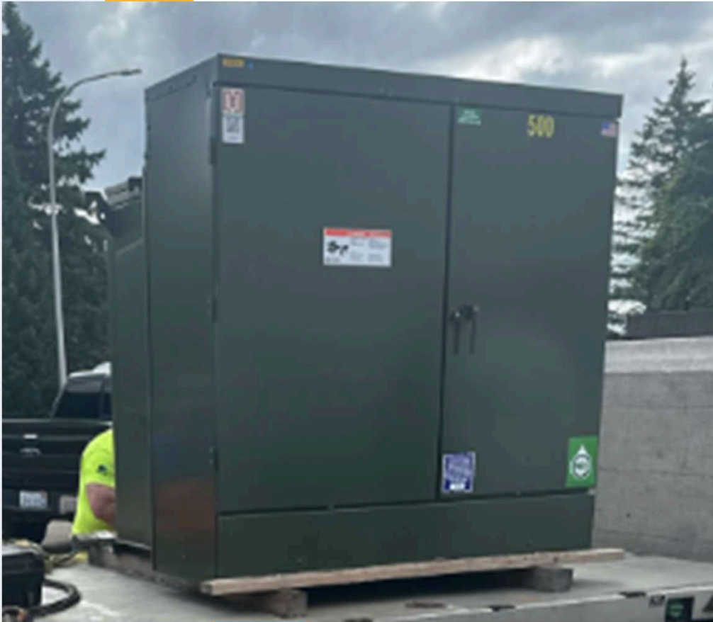
New Electrical Transformer for Pool
