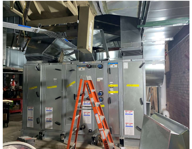
New Air Handling Equipment
