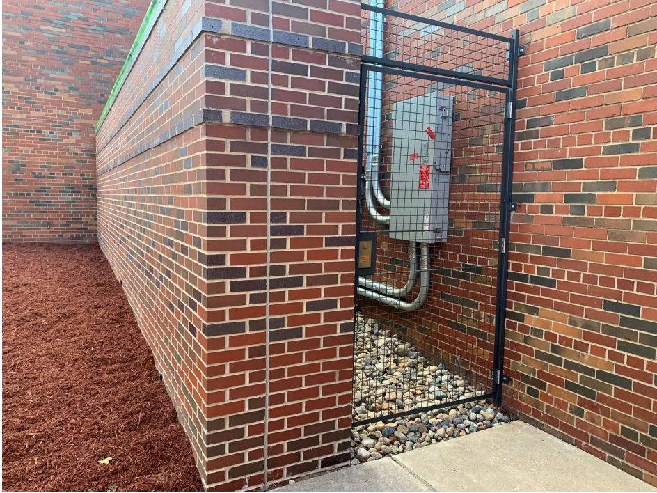
Pioneer High School Solar Array Equipment Screen Wall
