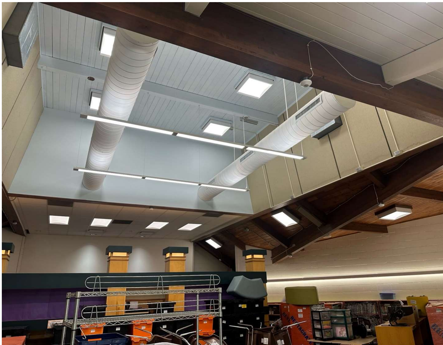
Lawton Elementary School – LED Lighting
