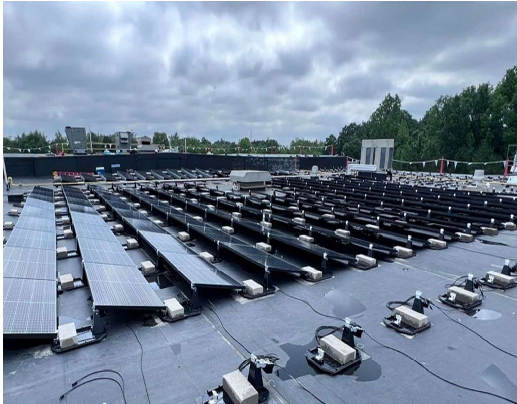
Scarlett Middle School —Solar Array
