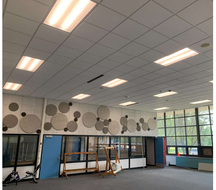
Air Conditioning & LED Lighting - Band Room
