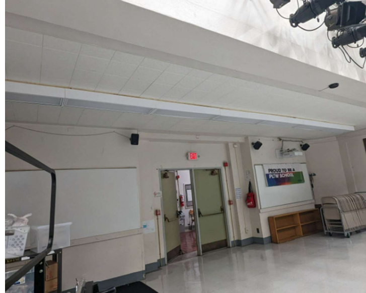
Angell Elementary - Additional LED Lighting Upgrades
