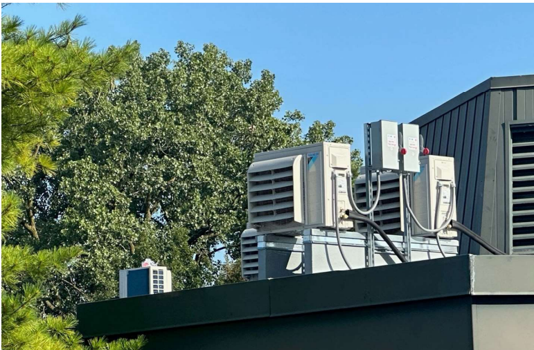
Lawton Elementary School – Air Conditioning
