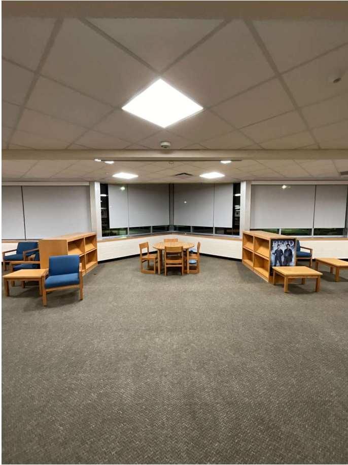
Air Conditioning & LED Lighting - Media Center
