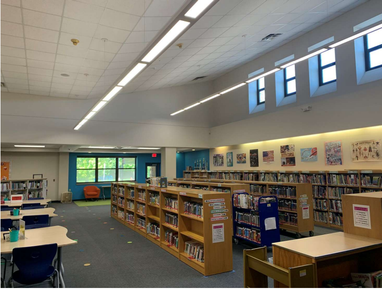
Ann Arbor STEAM – Air Conditioning & LED Lighting
