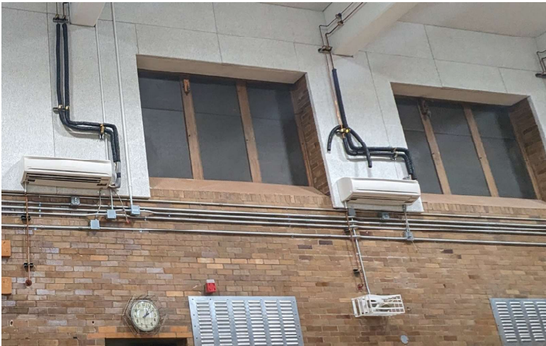
Bach Elementary School – Air Conditioning
