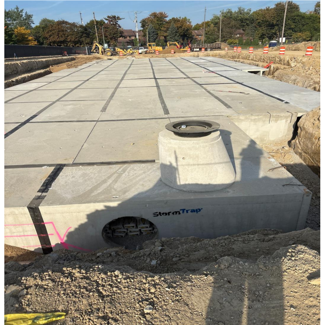
Underground Retention System
